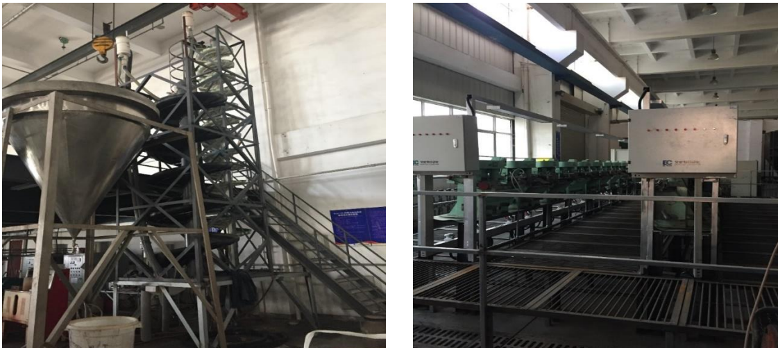
Figure 13: Hunan Research Facility spiral and flotation circuits
